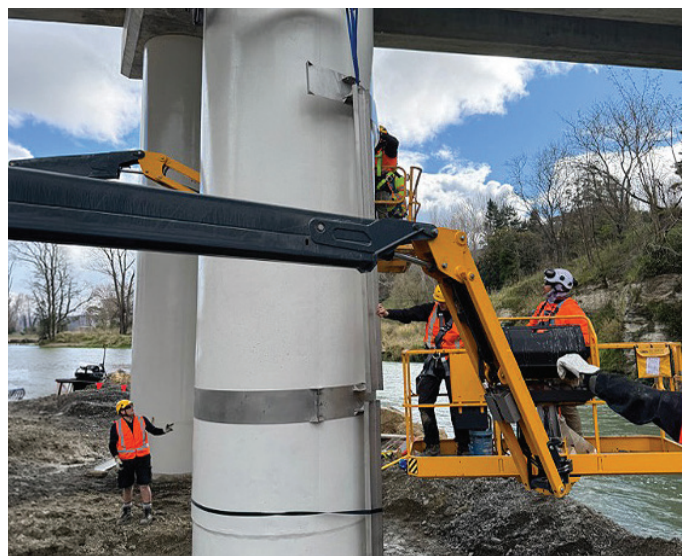
Telemetry Upgrades, Hawke's Bay
