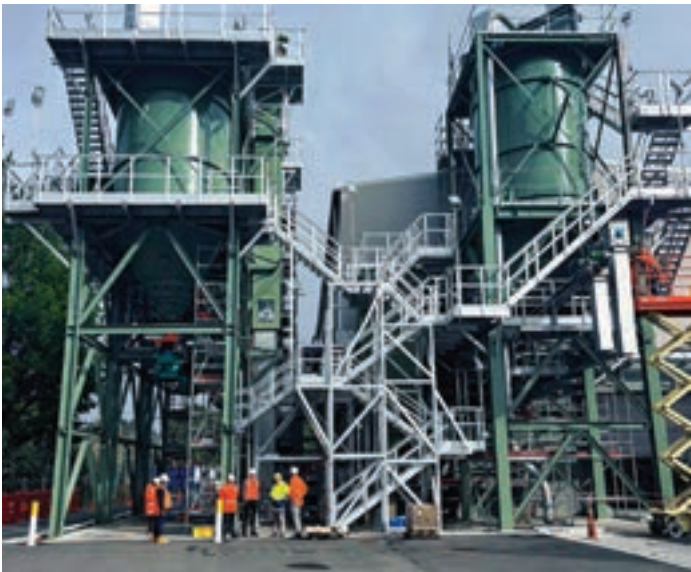
Thermal Drying Facility
