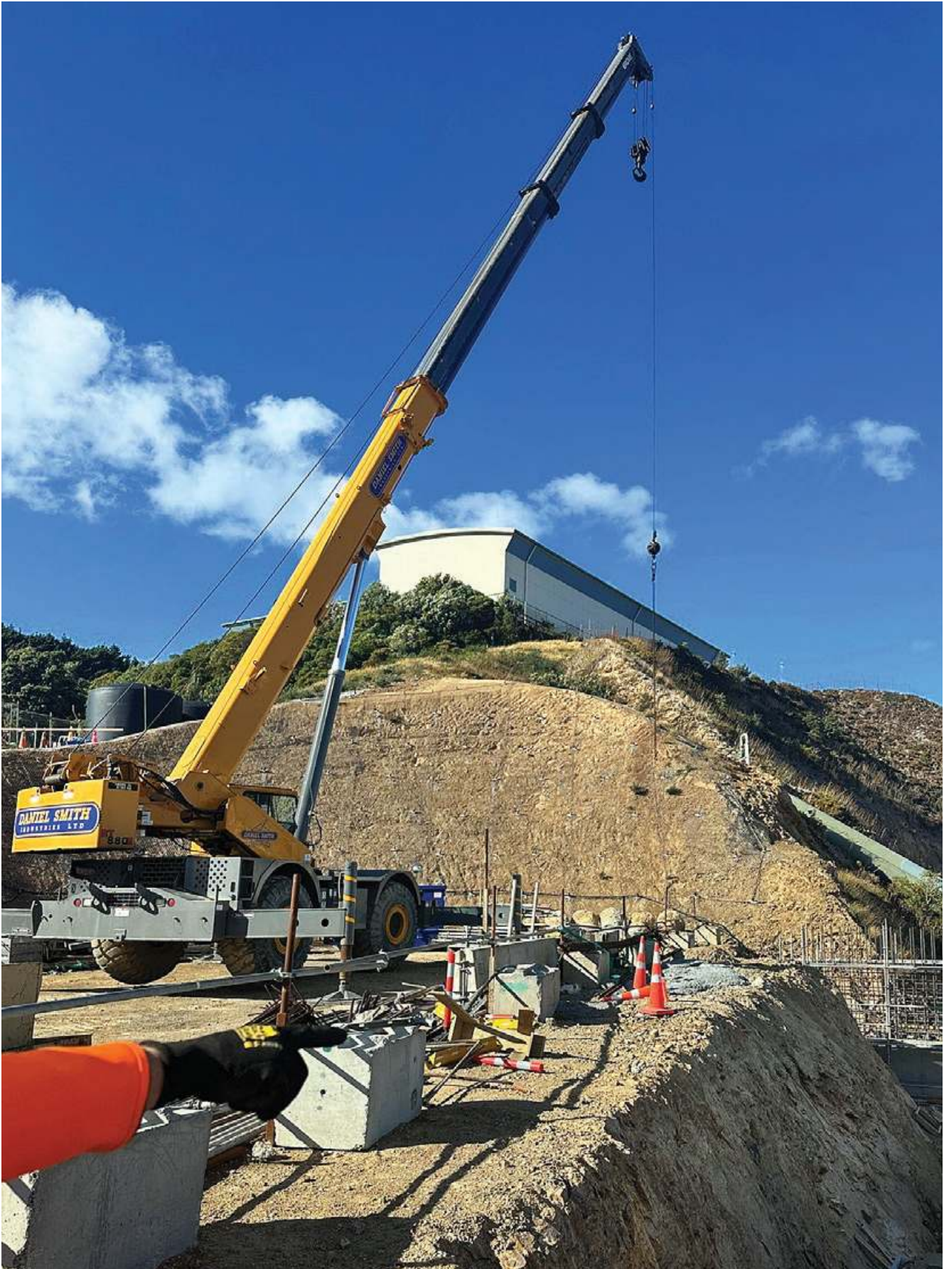
Wellington Sludge Minimisation Facility, Wellington – IFF Programme
