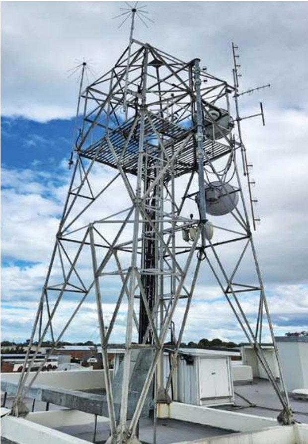
First LMR site built, Timaru
