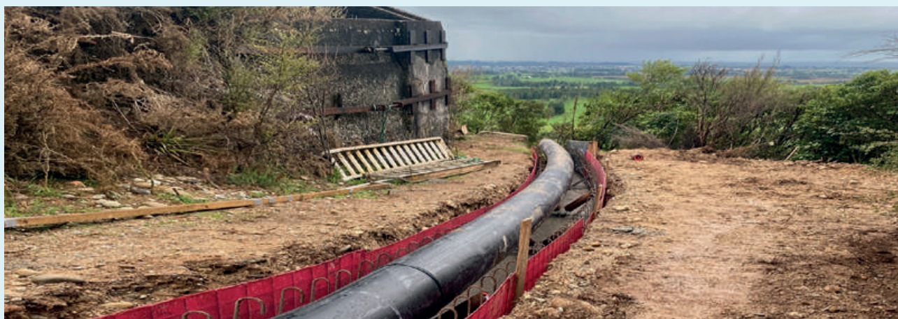
Westport trunk water main
