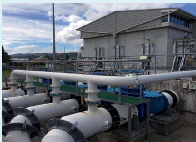
Gisborne Wastewater Treatment Plant
