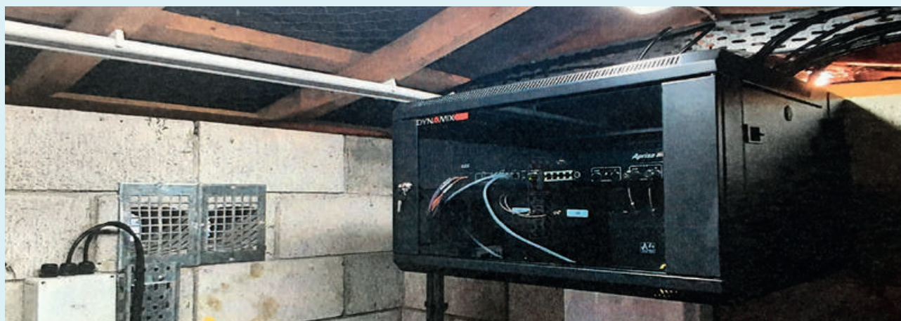
Taupo New SCADA installation at Hatepe
