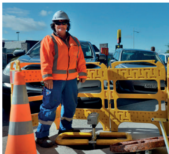
Sewer Line Rapid Assessment Tool in action in Taupō CBD.
