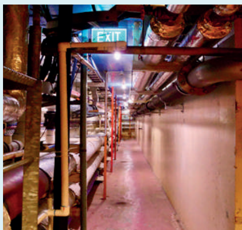
Palmerston North Waste Water Treatment Plant
