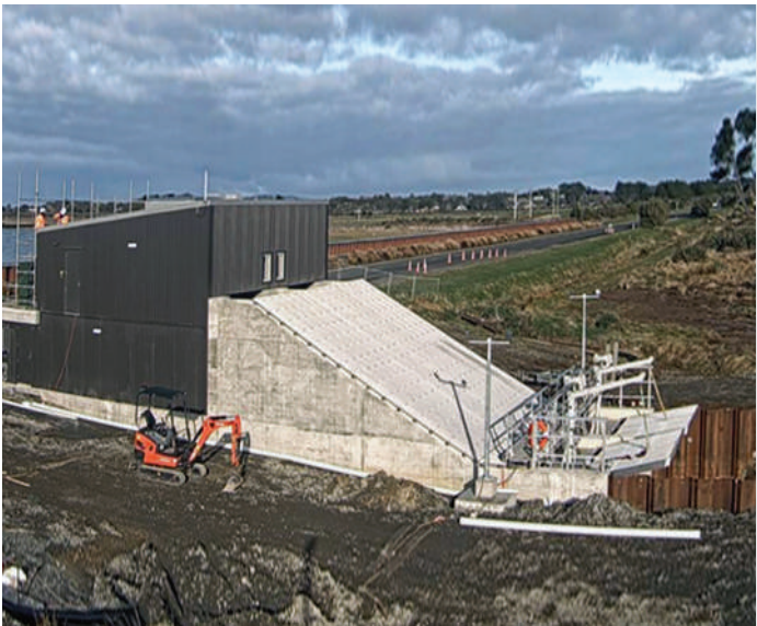
Stead Street Pumpstation
